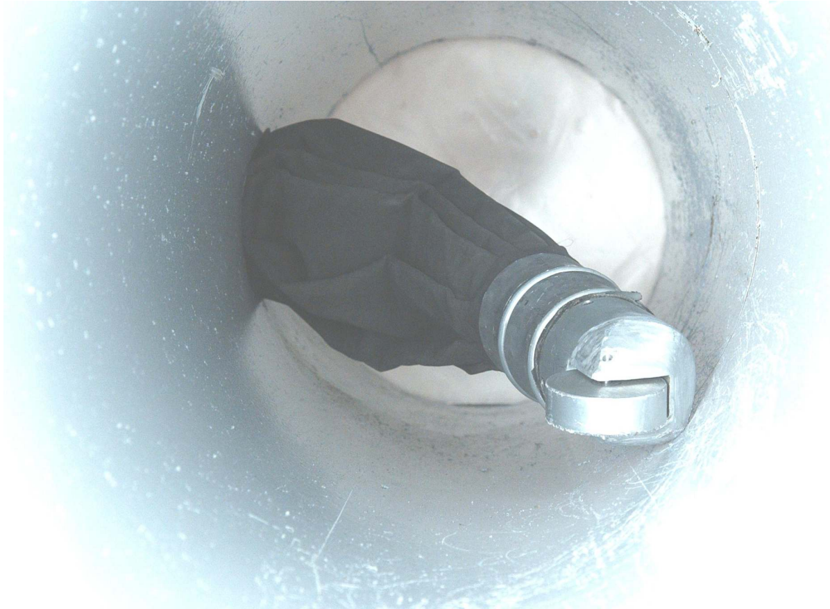
The MultiFlex Plug shown entering tapped pipeline
